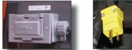
Figure 3-3. AC Outlet and Electrical Plug
